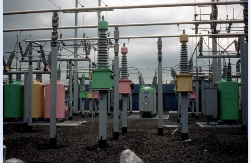
Viewland/Hoffman Electrical Substation, Seattle
